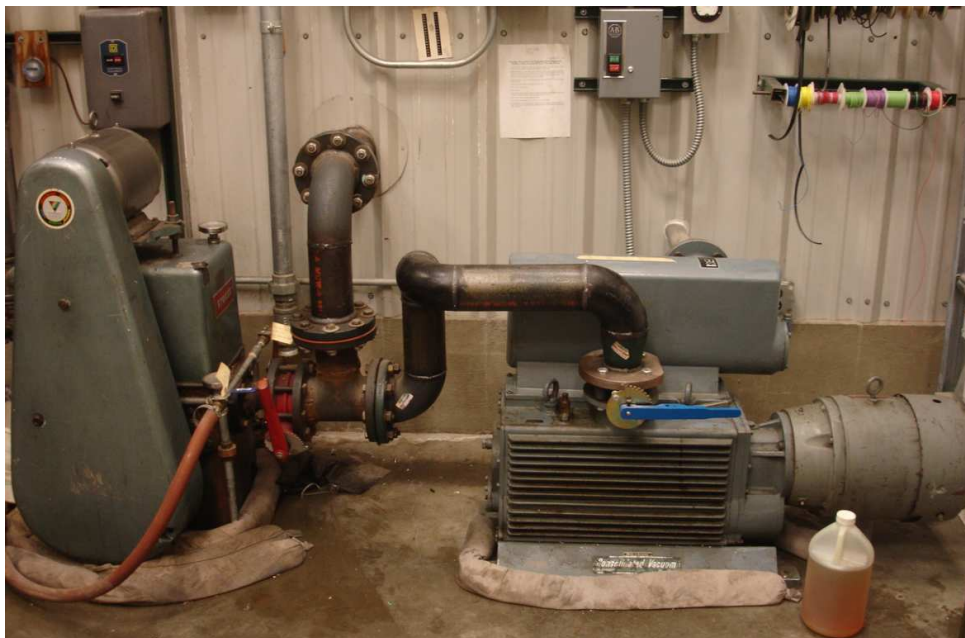
Figure B.7: PQFLT facility, vacuum pumps
