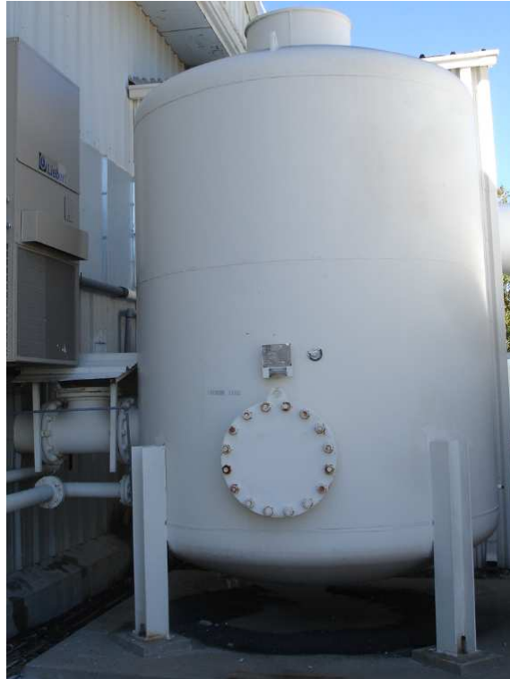
Figure B.8: PQFLT facility, vacuum tank
