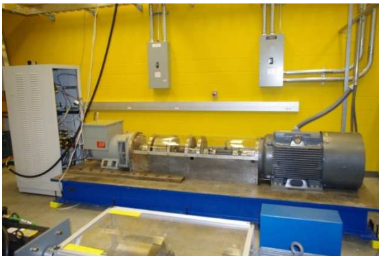
57 kW Main Power Generation Module (MPGM)
