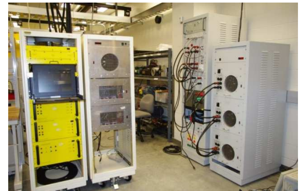
Zone 2 (left) and 18 kW Pulsed Power Load
